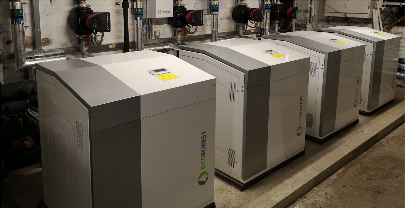
Four Ecoforest heat pumps in the Gatton Hall plant room
