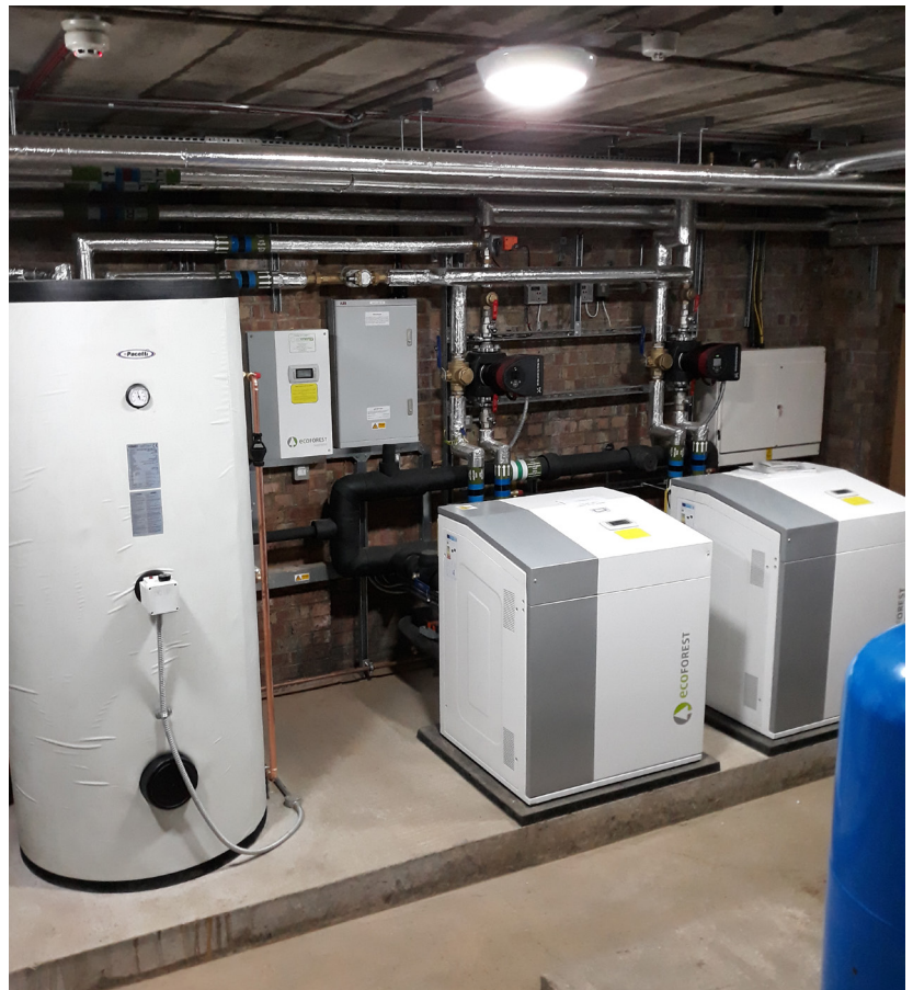
Each of the boarding houses has its own plant room connected to a shared ground array, either in the lake or using boreholes
